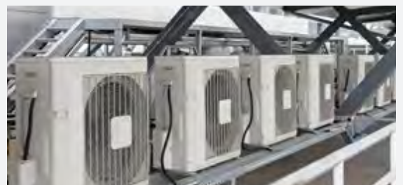
Outdoor Equipment of air conditioner
